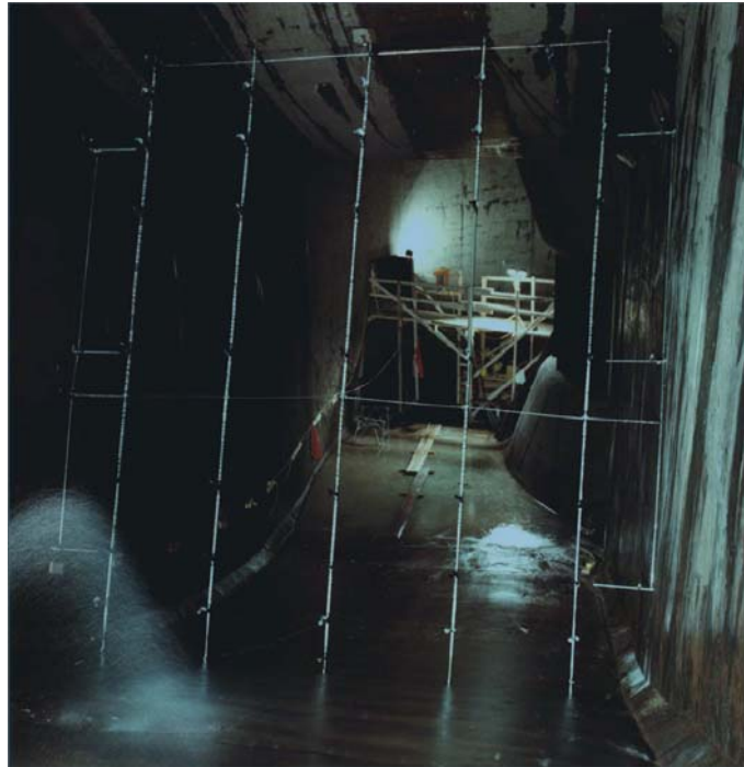
Figure 3 - Current Meter measurement Set up in a Penstock.
