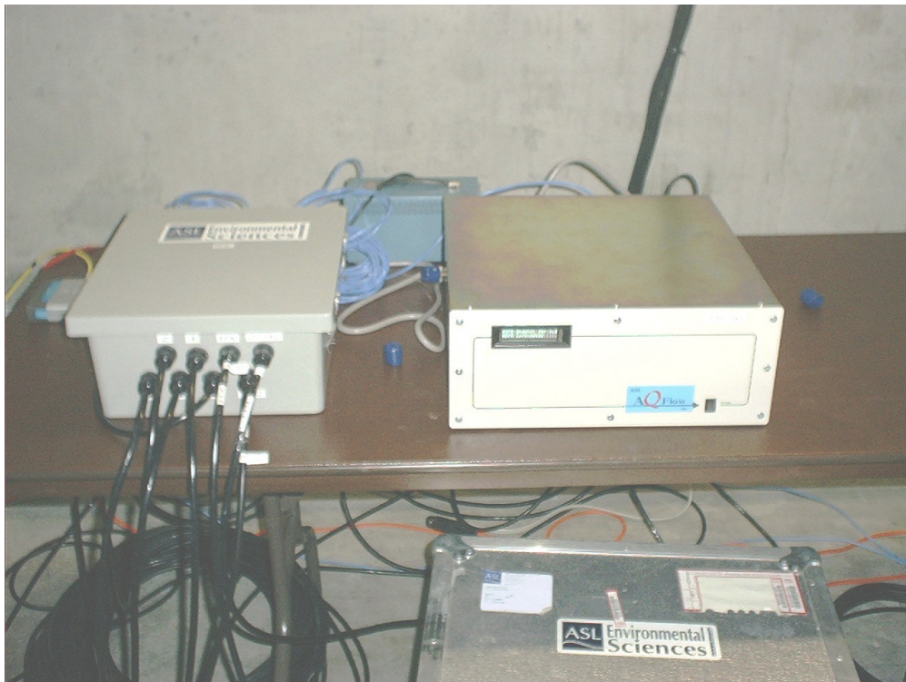
Figure 6: Monitor control unit and one switching box.
