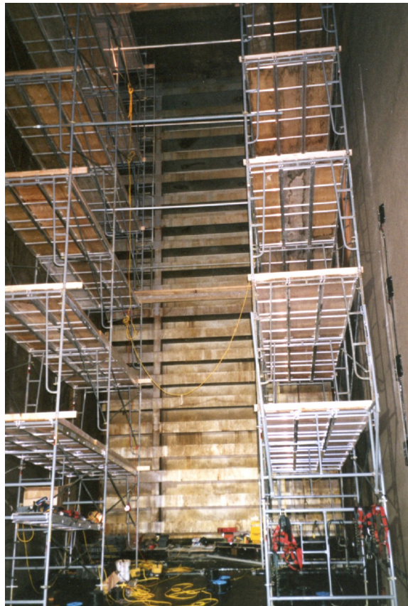
Figure 2: Interior of Bay A, Unit 4, during installation of the arrays and cabling.
