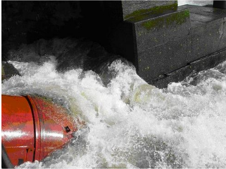
Fig. 2: Discharge from Unit 11 draft tube
